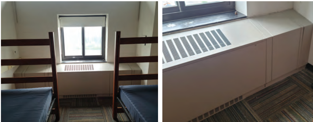
Examples of a fully assembled Carson Solutions FCE in a sample dorm room
